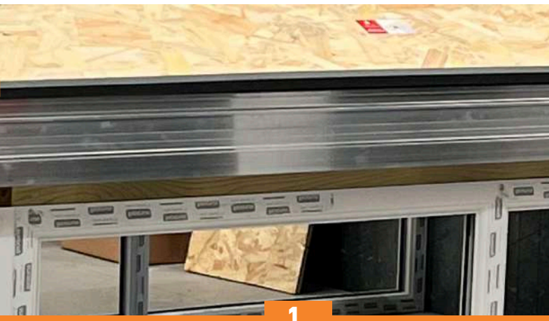
EAVES BEAM PACKING: THE SOFFIT EAVES WILL REQUIRE PACKING UP BY 45MM TREATED TIMBER.
